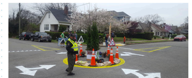
Volunteers install the TURBO traffic circle, with traffic control help from the Metro Police department.
